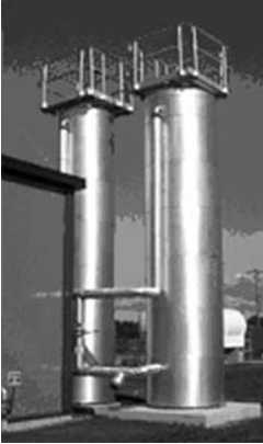
Picture 3: Sulfatreat® H 2 S-removal
